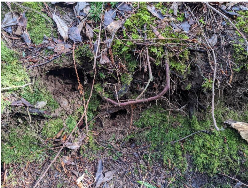
Figure 5 – Erosion of ditch bank
