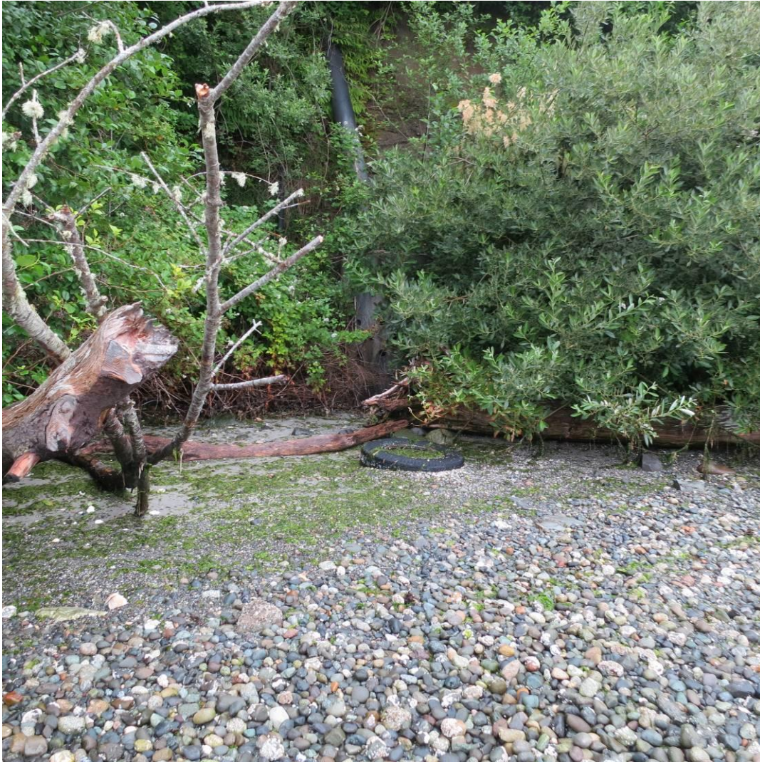
Pope Way Outfall – July 13, 2017 (Outfall Structure Behind Driftwood and Vegetation)
