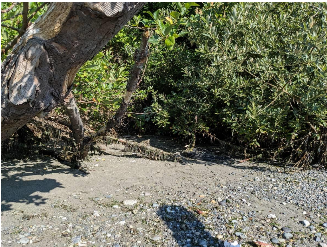
Pope Way Outfall – July 13, 2023 (Outfall Structure Behind Driftwood and Vegetation)
