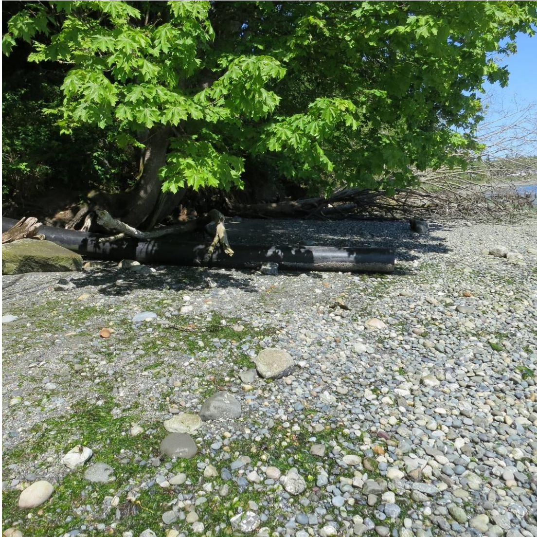
Montgomery Court Outfall (Between 70 and 120 Montgomery Court) – May 23, 2017
